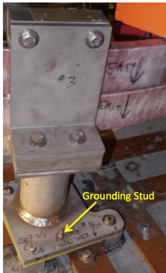
Figure 14 Bussbar floor support missing grounding jumper
