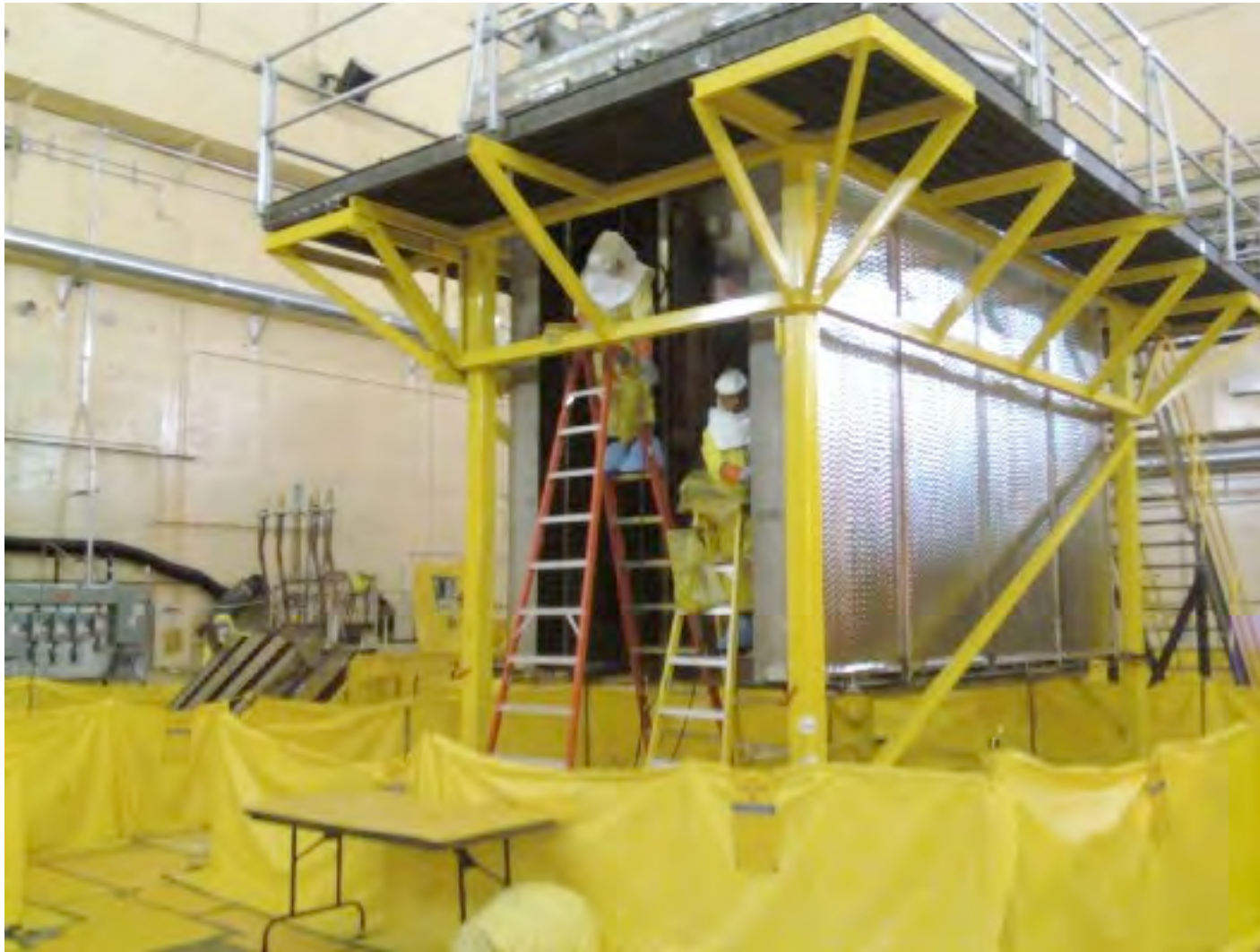
Hoods work well - cooler & cleaner
