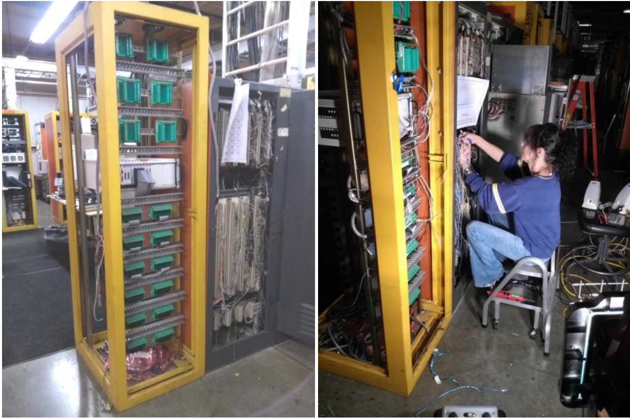
Local Control Center and wiring updated
