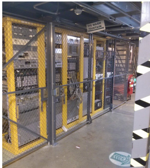
PLC Gallery Racks, Chassis, software, Cabling Completed
