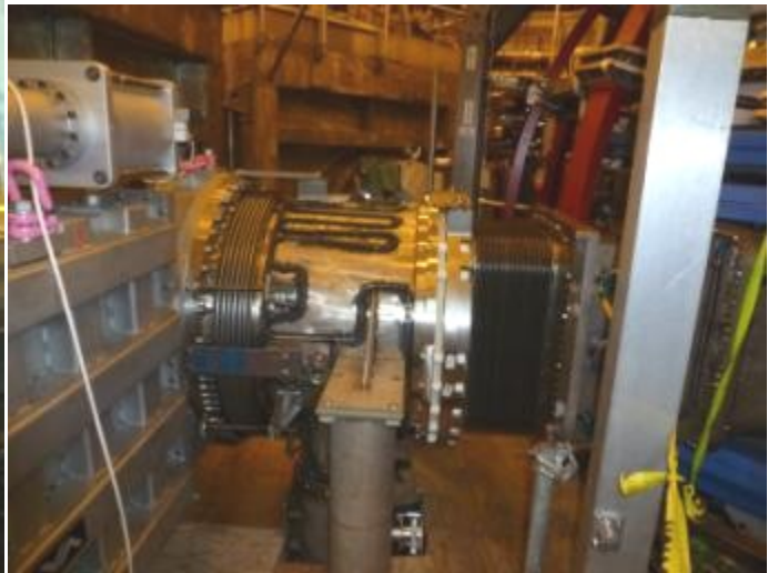
NBI Duct Installed
