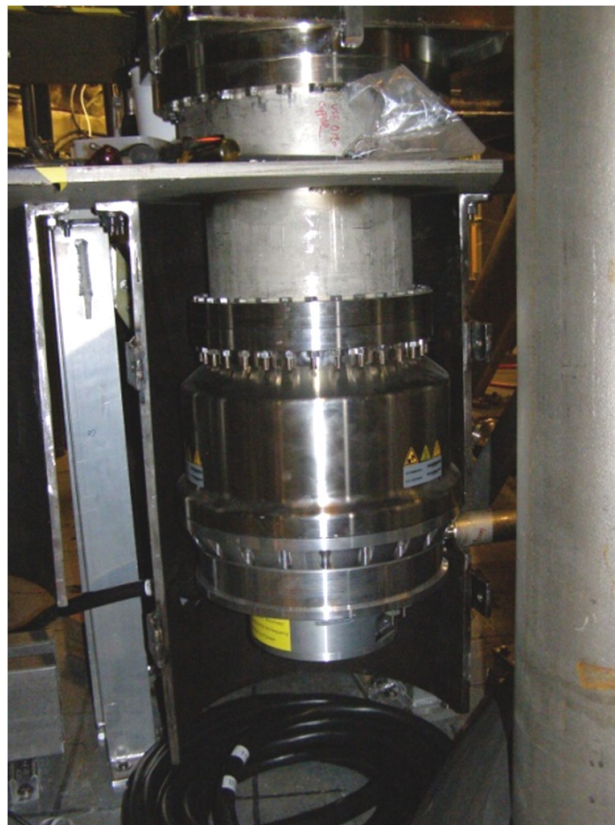
Torus Vacuum Pumping System Installed
