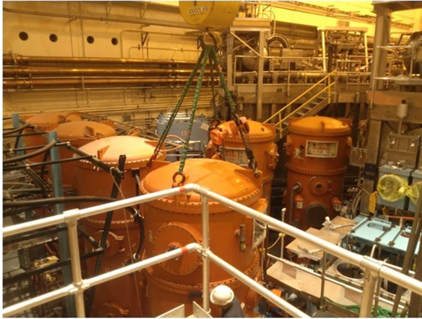
High Voltage Enclosures (HVE's) Relocated
