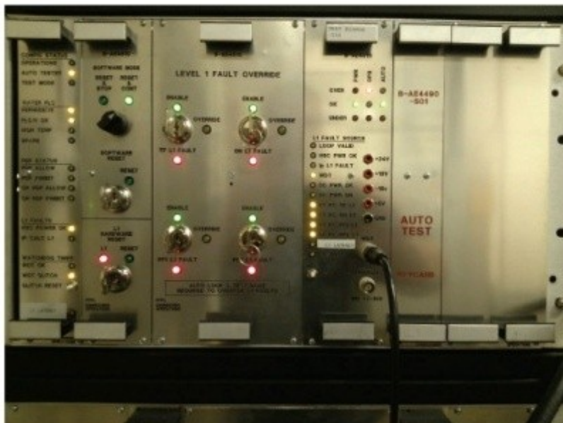
Junction area DCPS hardware user interface installed
