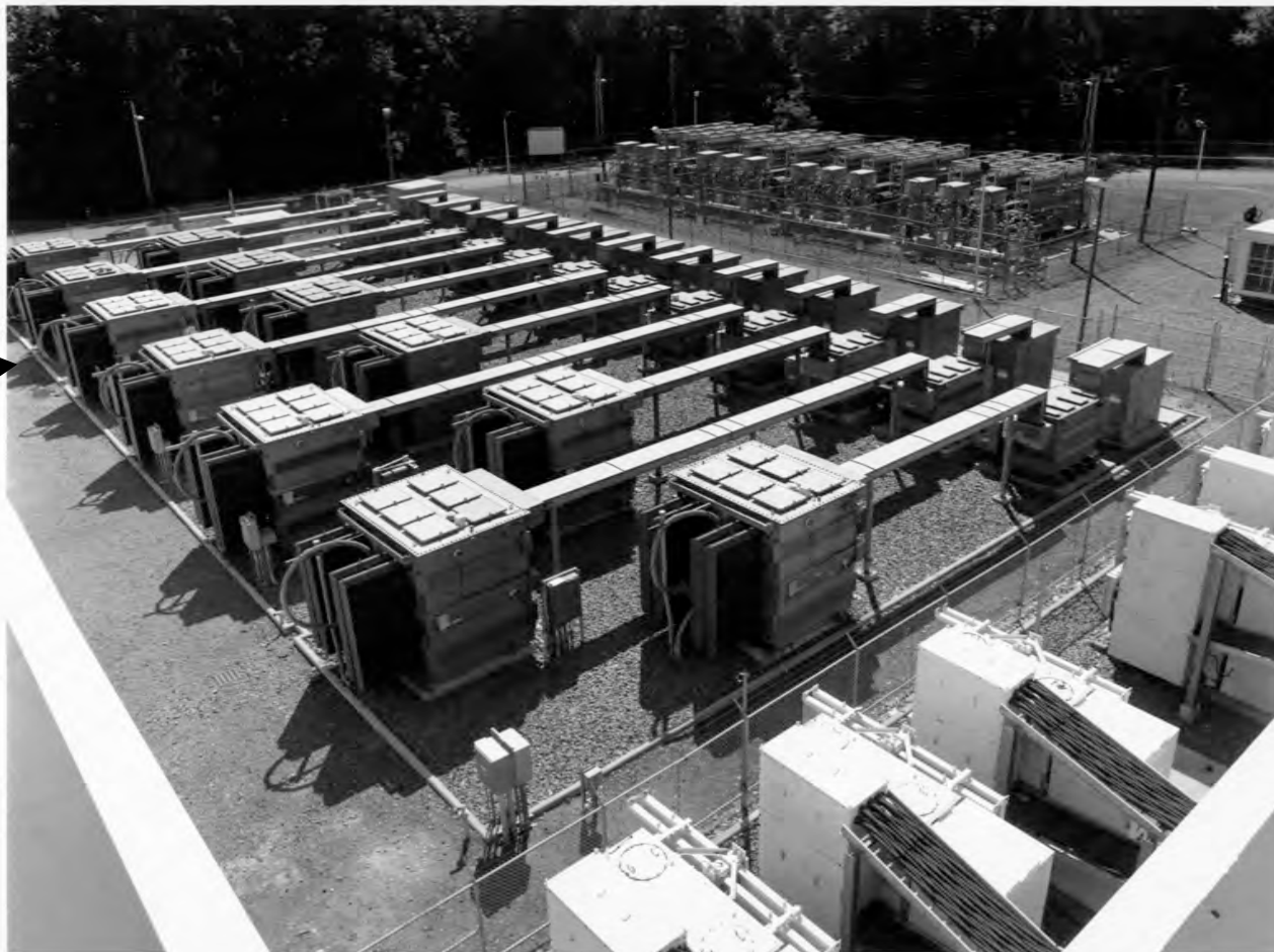
NBI NBPS Switchgear and Transformers
