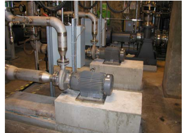
•New pumps for BL IS & ID DI water
