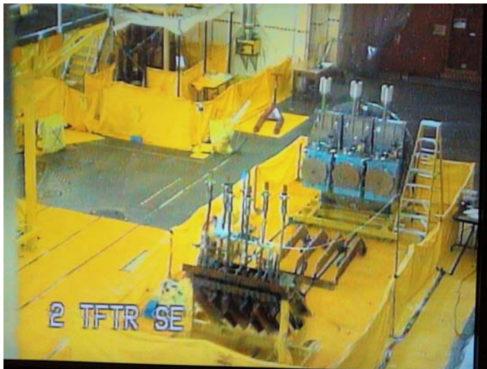
BL4 Magnet and 90 inch flange
