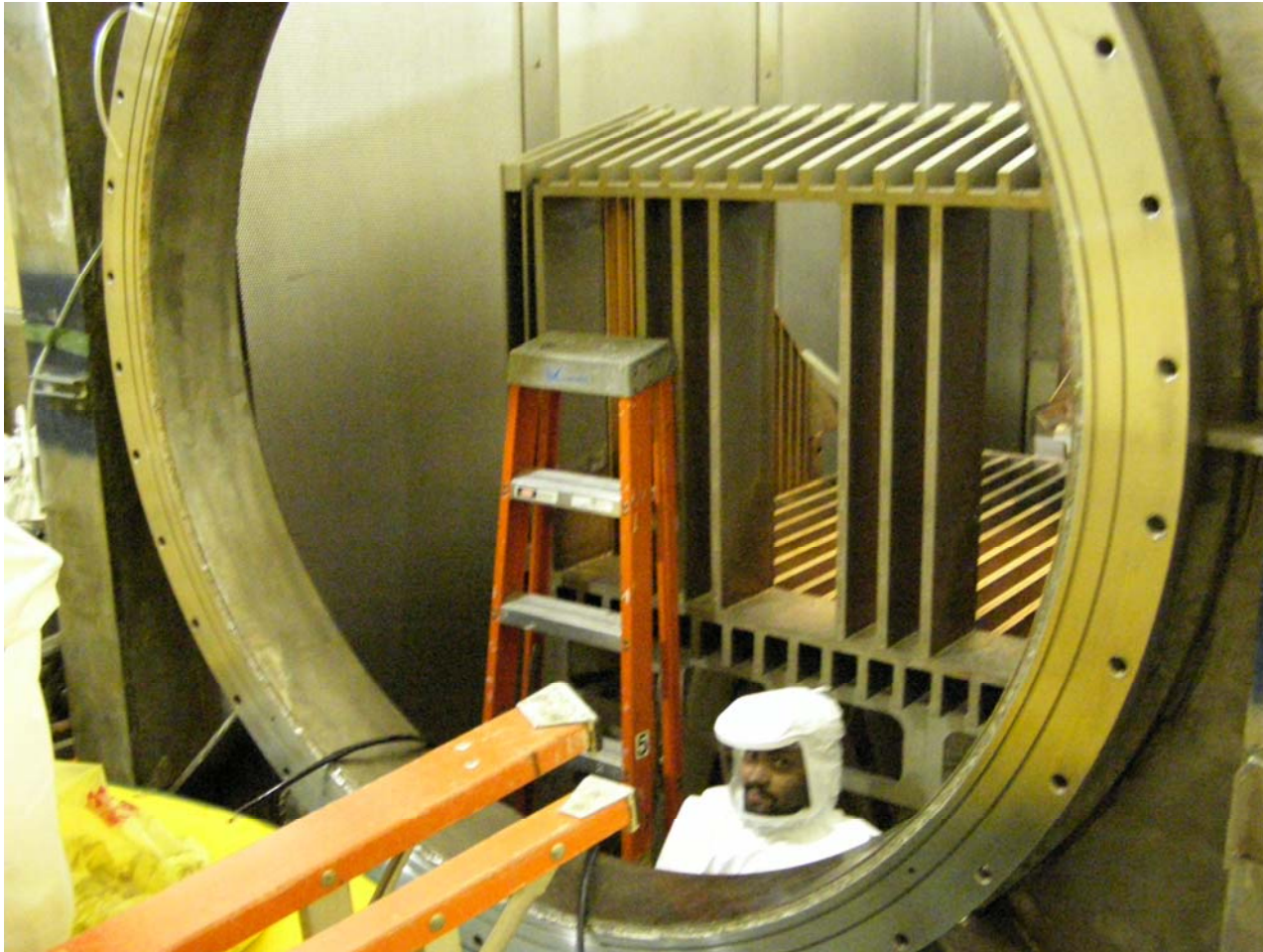
Hoods made BL entry possible and safe for decon wipedowns after use of sprayer
