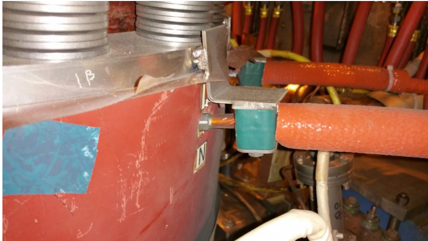
Figure 10.0-1 Coolant Tube Support As- Installed After the Arc Fault
