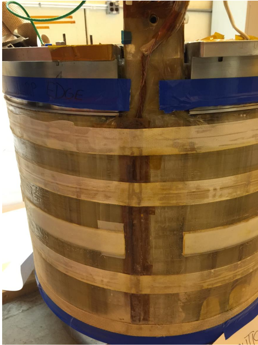
Figure 4.0-3 Photo of the Failed PF1a upper Coil after Removal and Before being sent for Radiography
