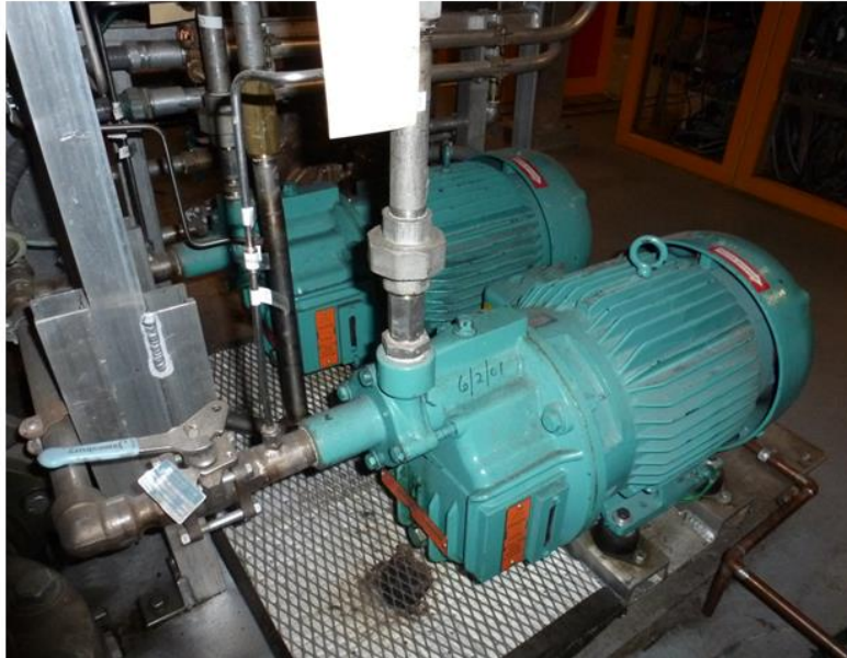
Figure 6.4-2 High Pressure Pumps Used to Supply Water to the OH, PF1a, b and c Coils
